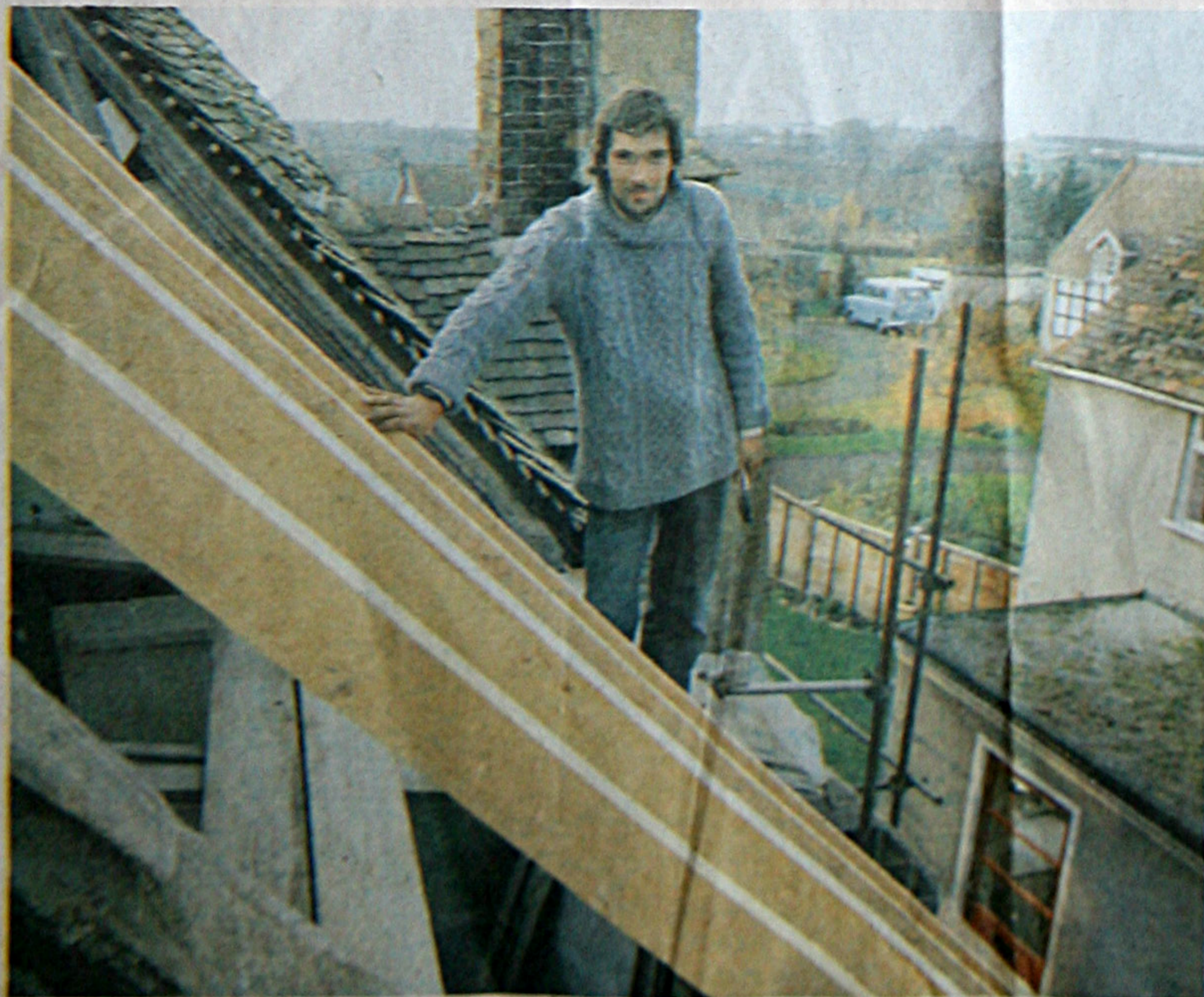
Workman Lyndon Bowley renovating the roof of the Vicarage Cottage in High Street.
